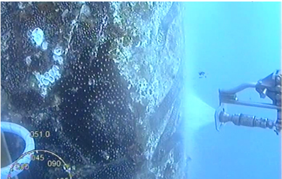
Dive Works robot and Toxfree water blasting to remove build-up from pipes underwater.
